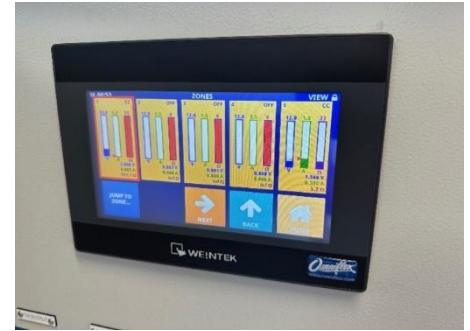
PowerView CP system close up
