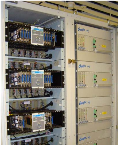
Some of the old and new annunciator systems during the change over process performed while the plant was still operational.
