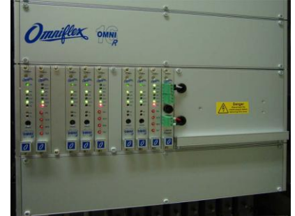
The Omni16R rack based alarm annunciator.
