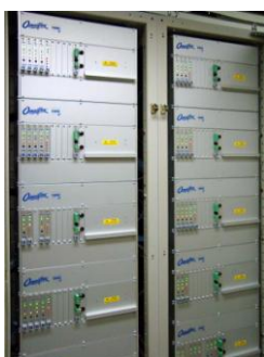
The new Omni16R Alarm System
