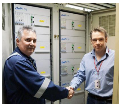
Geoff Roberts, Engineering Technician at Shell with Ian Southerton from Omniflex, during system handover.
