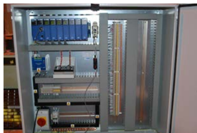
One of the Maxiflex alarm systems supplied by Omniflex.
