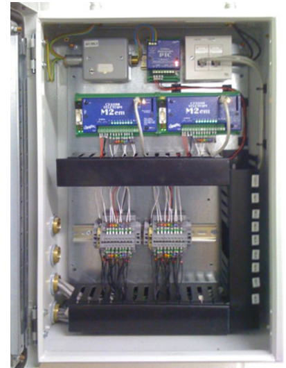
One of the local meter concentrator panels supplied by Omniflex.
