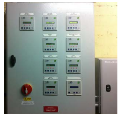
One of the hospital's existing sub-metering panels
